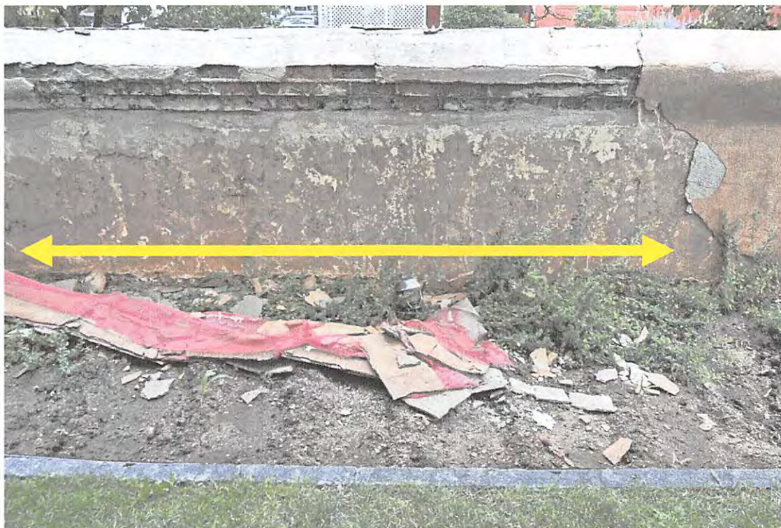
Figure 8: Example of failed stucco, north wall, interior, facing north.
