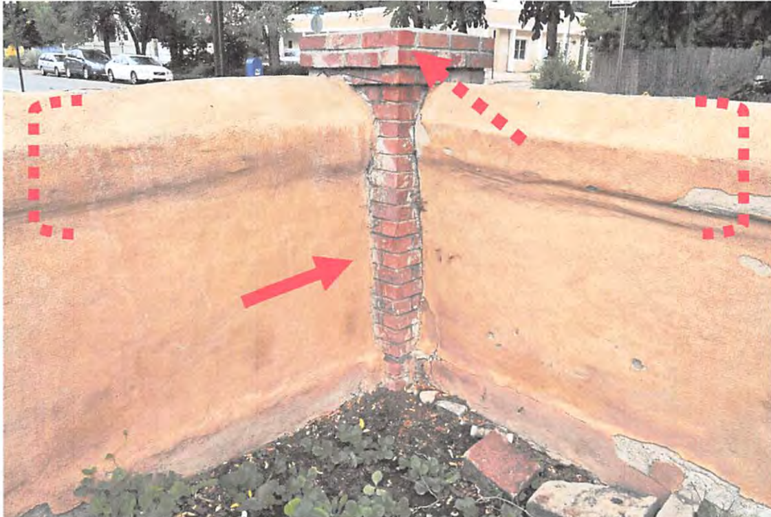
Figure 9: Northeast corner, interior, facing northeast. Dashed brackets indicate probable post-1964 creation of angled coping. Dashed arrow indicates additional non-historic courses of brick. Solid arrow indicates general change in design and loss of integrity through non-historic stucco applications.
