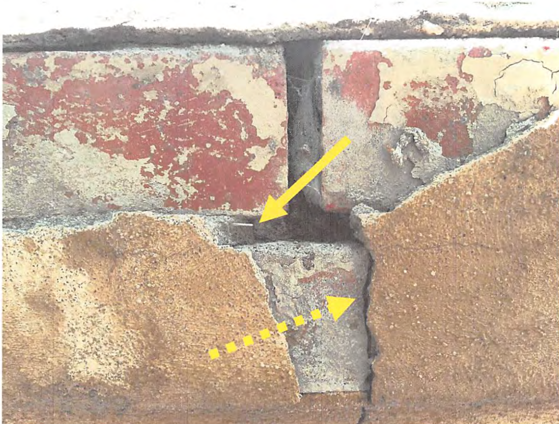
Figure 5: Brick construction under coping. Solid arrow indicates recent flex mesh reinforcement in mortar. Dashed arrow indicates the coping understructure lacks the earlier layers of plaster/stucco found on the planar portion of the wall below.
