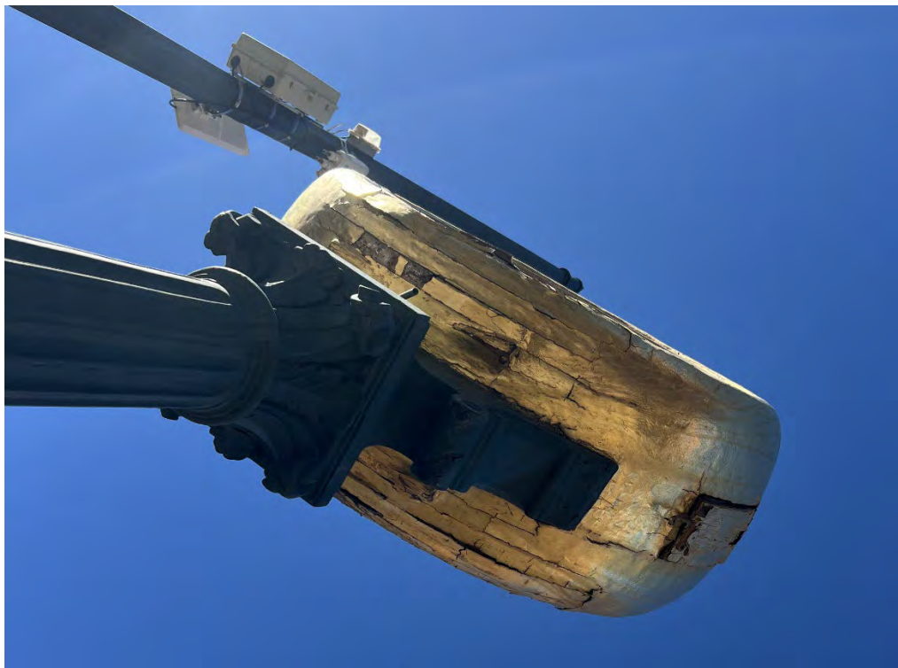
Photo 12. Detail of damage to clock face, view looking up from northwest corner. (July 2026)
