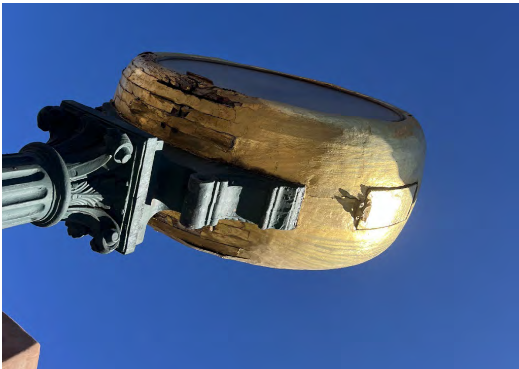
Photo 10. Detail of damage to clock face, view looking up from southeast corner. (July 2026)
