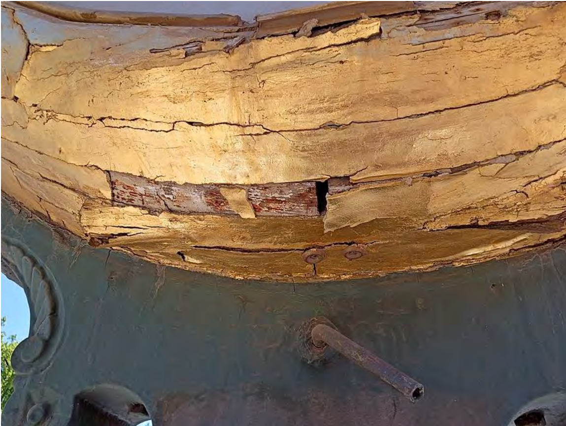
Photo 9: North elevation casing, advanced deterioration. Camera facing up.
