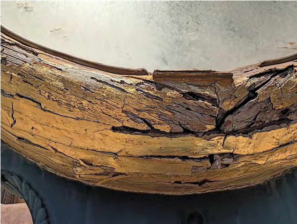
Photo 8: South elevation casing, advanced deterioration. Camera facing up.
