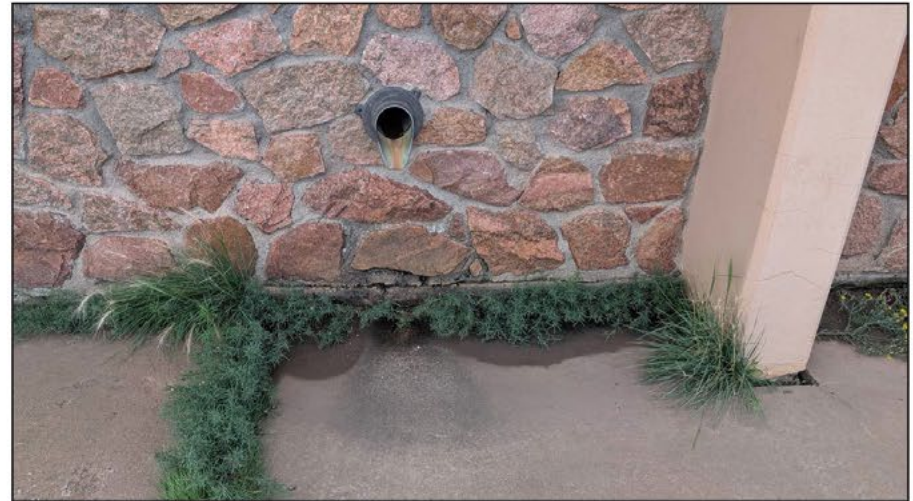
1) Roof Water Infiltration into Building Foundation
