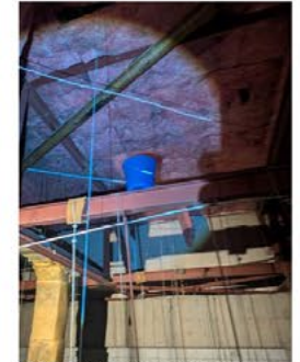
2) Leaking Roof Drain
