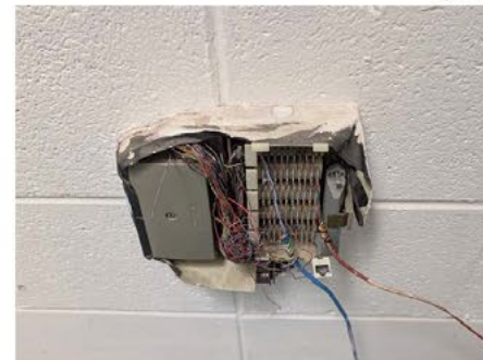
3) Telephone Equipment, Office 147
