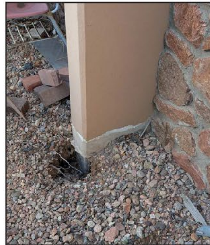
4) Exposed Building Foundation
