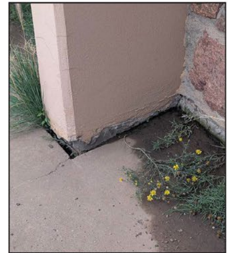
5) Settlement of Exterior Slab
