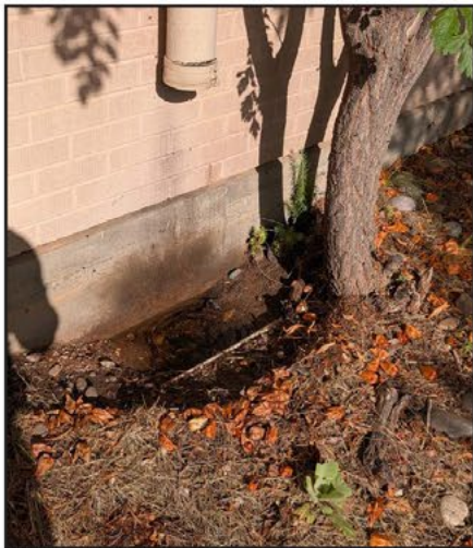
2) Roof Water Infiltration into Foundation
